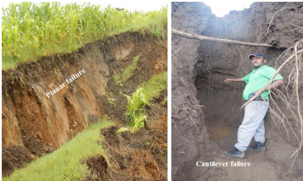
Figure 2. Pictures illustrating dominant types of bank failure observed in the Debre Mawi watershed; the left photo is of the study gully and the right photo is a headcut of a nearby gully located at a distance of 50 m.
